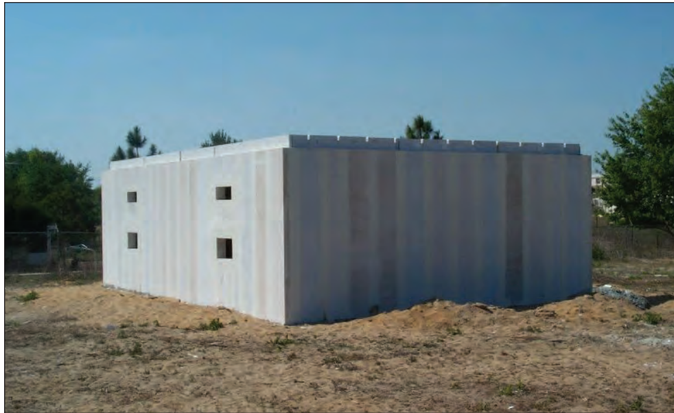
This 900 square foot communication equipment building shell made of AERCON wall and roof panels was built from start to finish in 8 hours.
